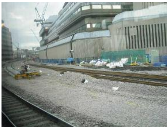
View of the southern approaches this month, with track laid, ready to be slewed over at Christmas
