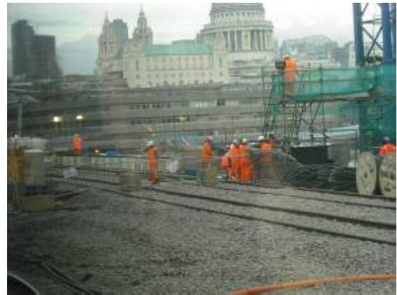
Poor view from passing train of the new platforms, taken in December 2010
